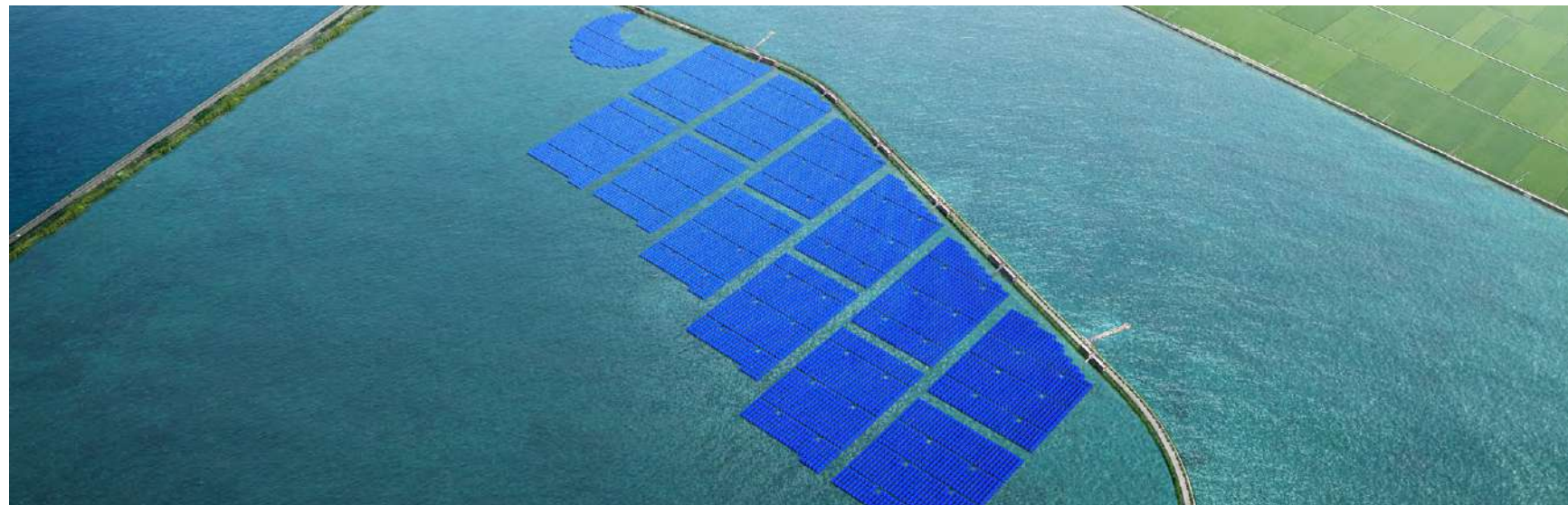
Goheung floating solar power plant
