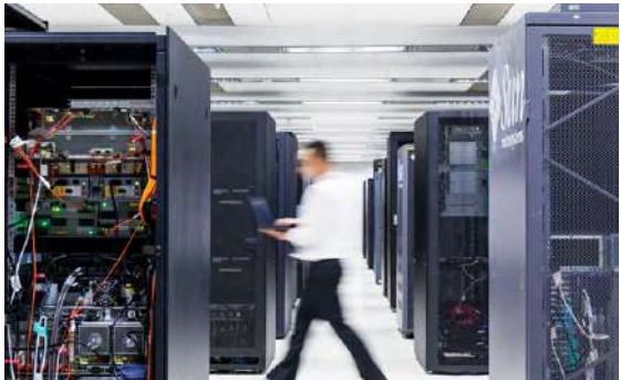
ICT big data center
